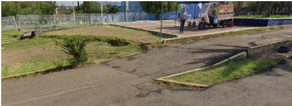
Fissured and ramped roads and ground due to surface faulting (©INEGI 2020)
