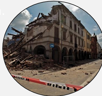
Collapse in Concordia sulla Secchia (Modena) after the earthquake of May 20, 2012 (DPC)
